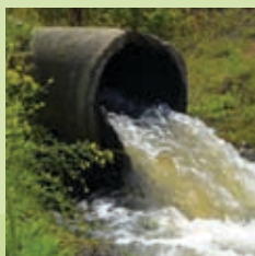
AFFORDABLE FIX FOR SEEPING SEWAGE...5
